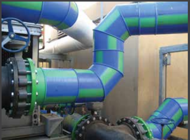
Los Angeles County Metropolitan Transportation Authority, Los Angeles, CA. 28-story chiller pipe retrofit.
