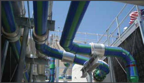
Bogle Vineyards, Clarksburg, CA. Chiller lines serving fermentation vats.
