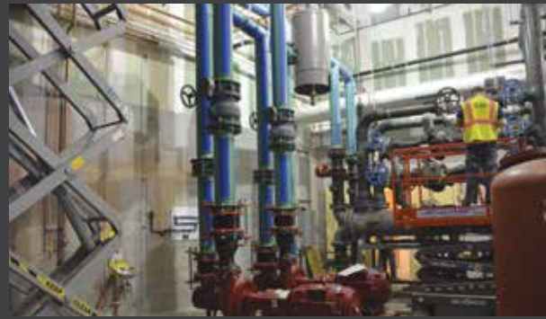
TCF Bank Stadium, Minneapolis, MN. Radiant field heating.
